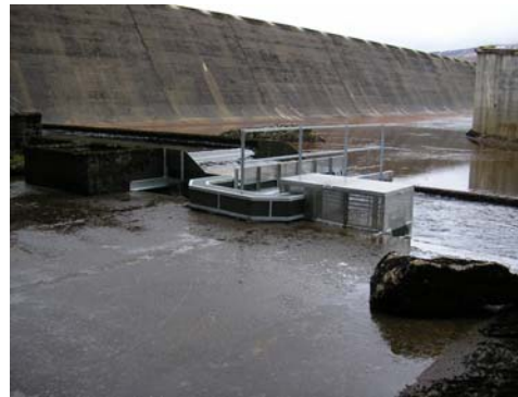
Figure 2b: New smolt trap installed at Alcan smelters, Spey dam. (A2Spey04).
