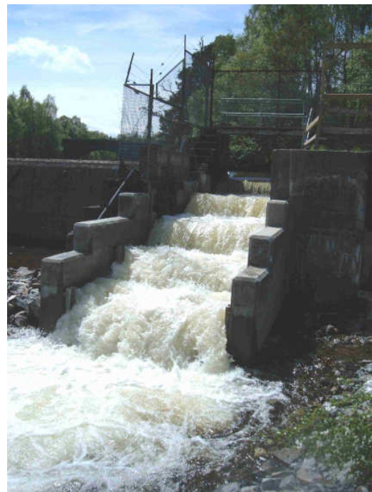
The new fish pass under construction at the Ceannacroc heck, River Moriston
